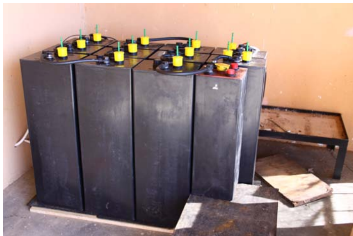
12 cells of 2 Volt each. Resulting into a total of Volt, with 1600 Amps. Each cell weights 145kg, so its 1.7t in total!!! The smaller cell at the very front still has to be exchanged, as the cell that was delivered was faulty.
