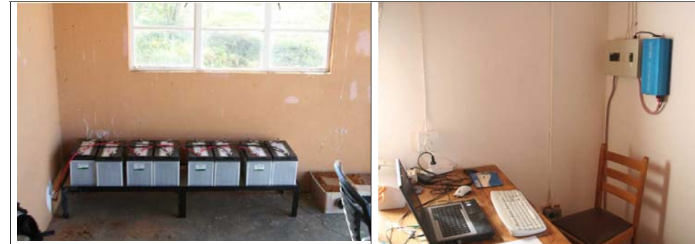
The solar panels charge solar batteries on the veranda of the research station. These are connected to the blue inverter on the wall of the research room that changes 24V to 220V. From here power plugs in every room of the house are powered, such as the white one on the left hand side of the picture that runs one of the two new laptops.
