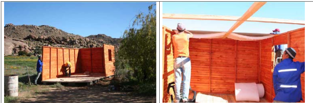
Building up the Wendy House was not so easy. We put some insulation under the roof to avoid it getting too hot in summer.
